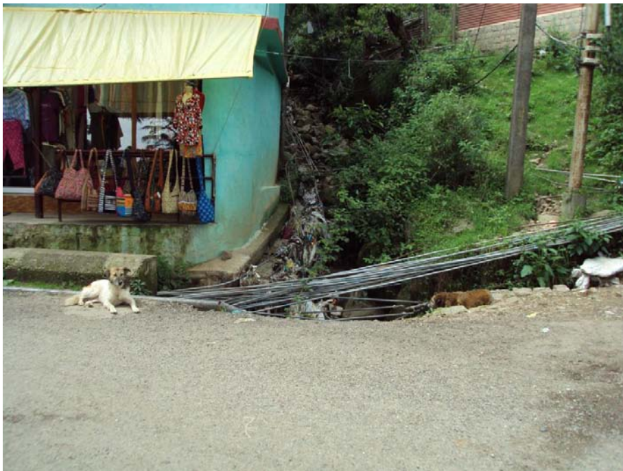
Figure 8: Multiple Pipelines along Road-sides suspended on top of Storm-water Drains
