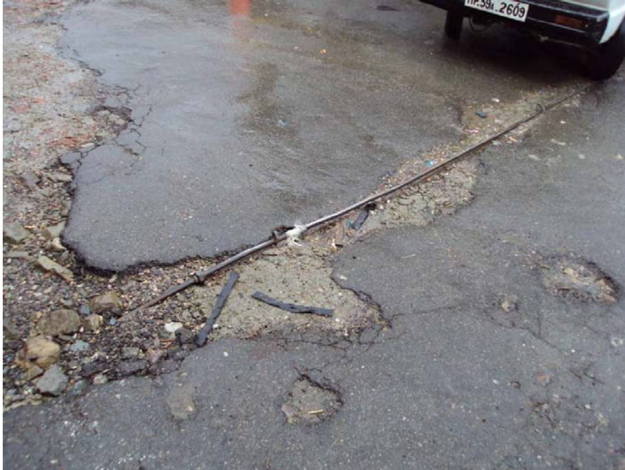
Figure 7: A Leaking Pipe with Plastic Taping
